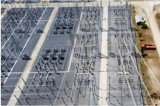
Electricity Station, Phuket Province
