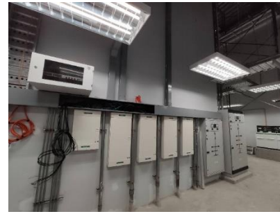
Electrical control panels
